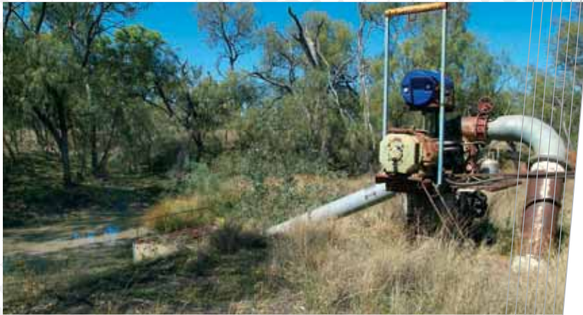
> Pump station on the Condamine River, Qld (MDBC)
