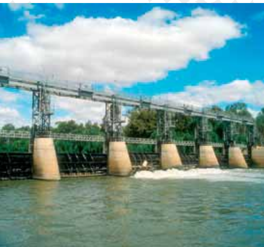
> Gogeldrie Weir on the Murrumbidgee River east of Darlington Point, NSW (CSIRO)
